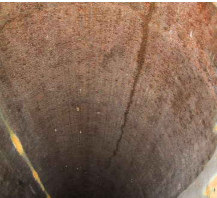
Picture of riser joint after displacement
